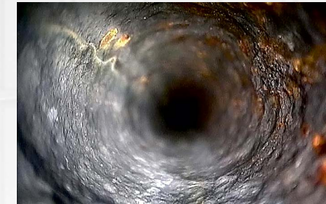
Real-Life Problem 2 Corrosion of Piping
